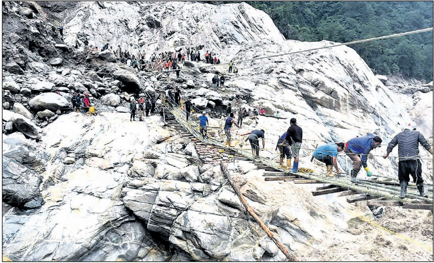
A temporary bamboo bridge being constructed at Chungthang connecting it to Pegong days after flash floods, in Mangan district, Sikkim
