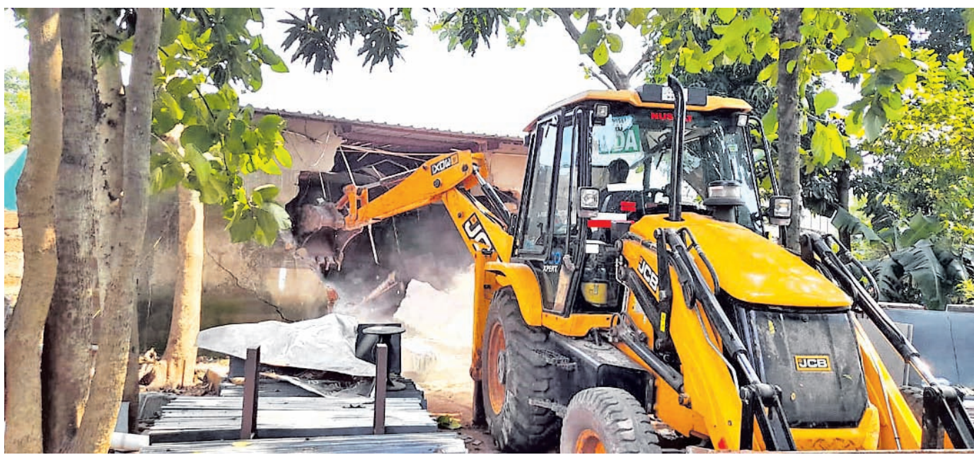
EVICTON DRIVE: An excavator deployed by BDA razing down an illegal construction at Patia in Bhubaneswar, Monday
