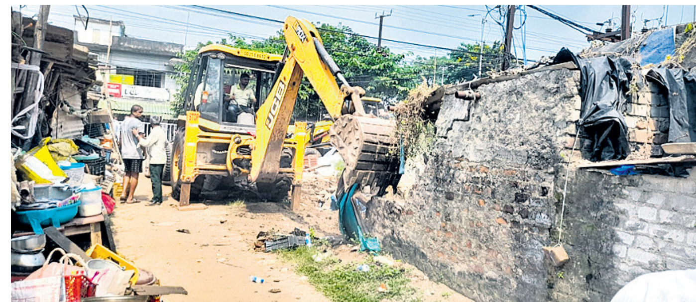
ANTI-ENCROACHMENT DRIVE: An excavator deployed by BDA razing down unauthorised constructions at Brahmeswarpatna in Bhubaneswar, Thursday OPPHOTO
