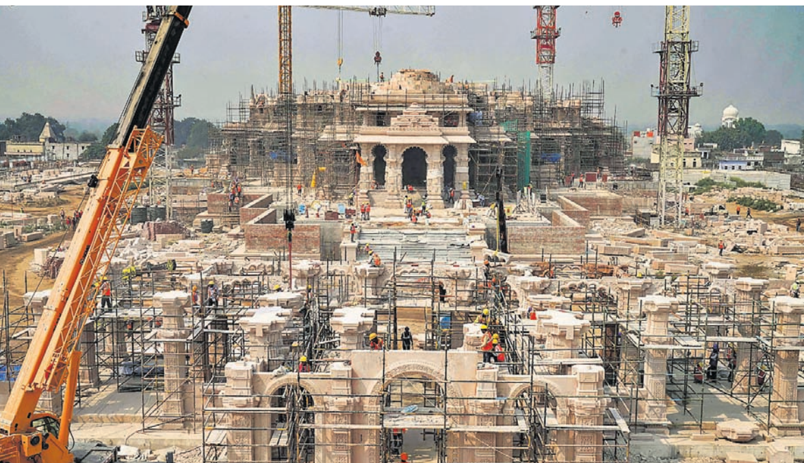
Labourers work at the construction site of the Shri Ram Janmabhoomi Teerth Kshetra, in Ayodhya, Uttar Pradesh
