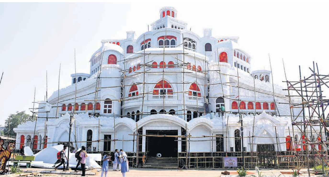
PUJA PREP: The Durga Puja pandal in Saheed Nagar area of Bhubaneswar is nearing completion, Monday
