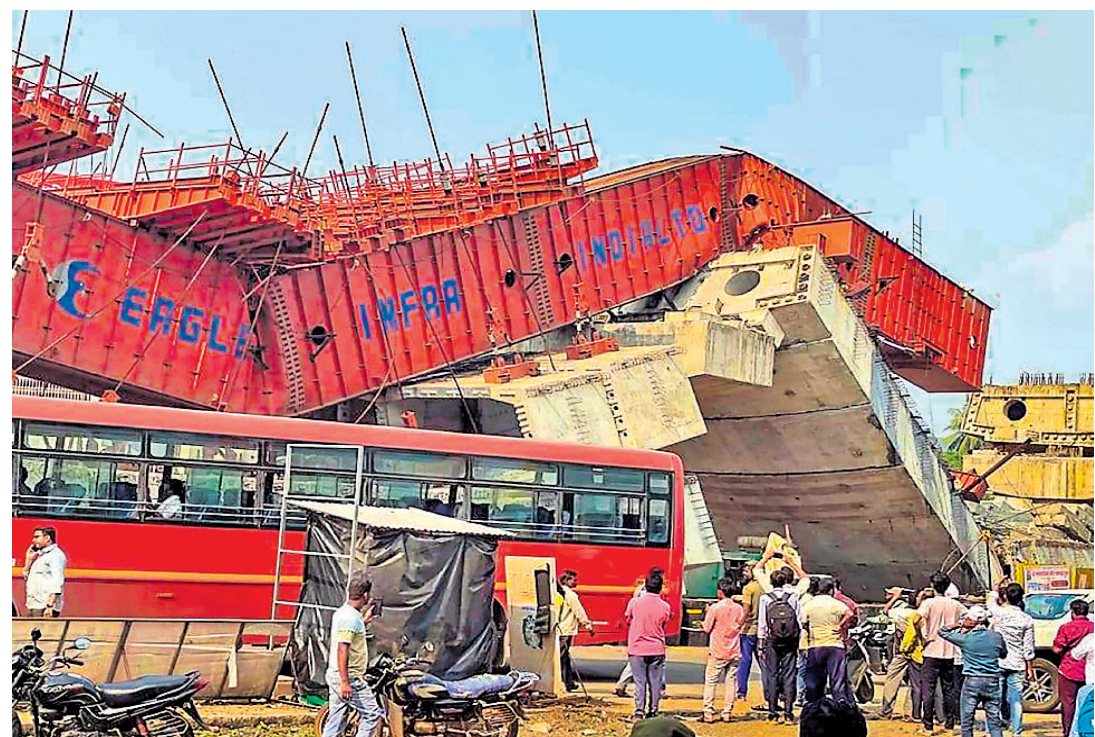
Locals at the site after an under-construction flyover on the Mumbai-Goa highway collapsed, at Chiplun in Ratnagiri district, Maharashtra
