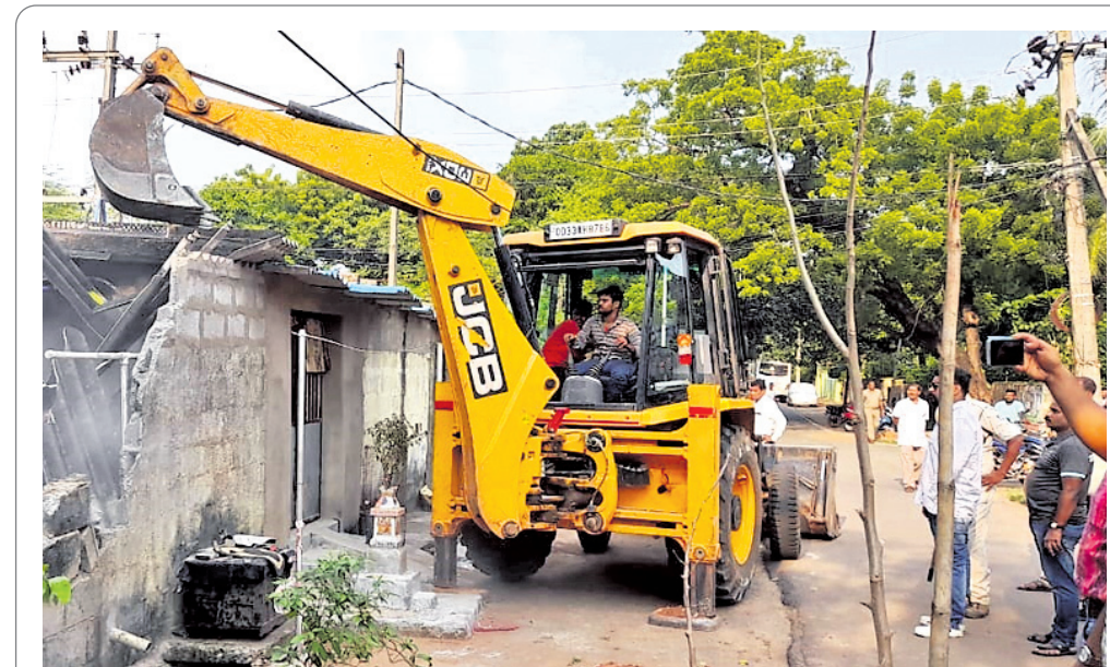
RAZING DOWN: An excavator engaged by BDA pulling down unauthorised constructions in Unit VIII area of Bhubaneswar, Monday
