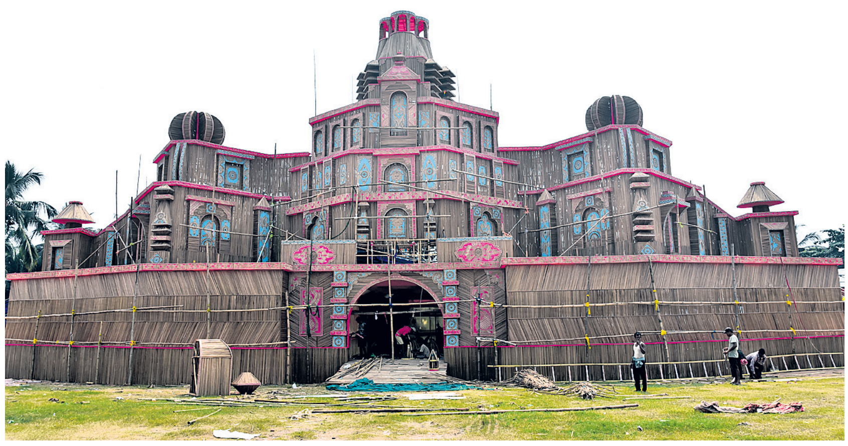
STANDING TALL: A replica of Thailand Buddha Temple being erected by Baramunda Durga Puja Committee in Bhubaneswar is nearing completion
