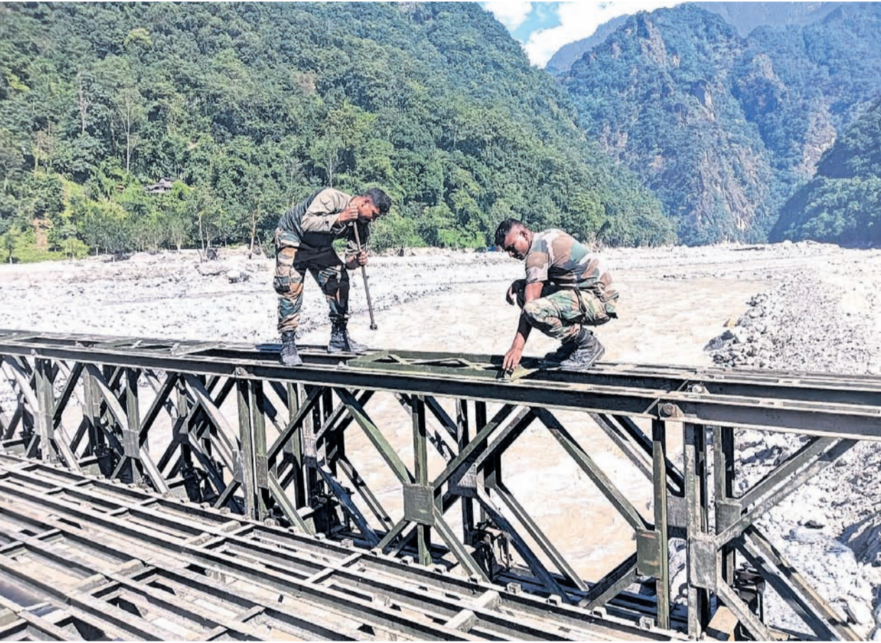
Troops of Indian Army with BRO and assistance of civil administration during an operation to reconnect North Sikkim through the first Bailey Bridge during flood, in Mangam, Sikkim
