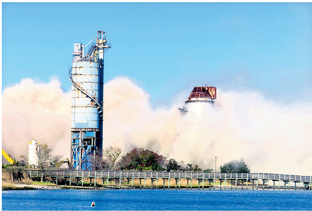
Debris and dust fill the air after smokestack at the former B.L. England power plant in Upper Township, N.J., was felled during a control demolition. The site will be redeveloped as a mixed use residential and commercial project, and a nearby electrical substation will be used to connect New Jersey's soon-to-come offshore wind farms with the electrical grid
