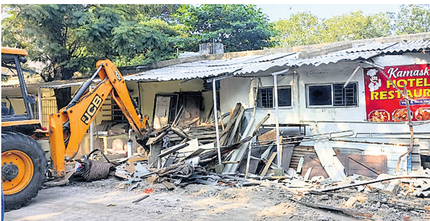
DEMOLITION DRIVE: An excavator deployed by BDA removing illegal constructions at Keshari Nagar located backside of Odisha State Secretariate in Bhubaneswar, Thursday
