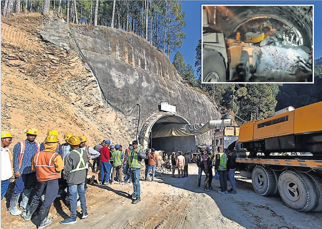
TRAPPED IN TUNNEL: Rescue and relief operations underway Monday after a portion of an under-construction tunnel between Silkyara and Dandalgaon on the Brahmaputra-Yamunotri national highway collapsed trapping 40 workers inside, in Uttarkashi district of Uttarakhand
