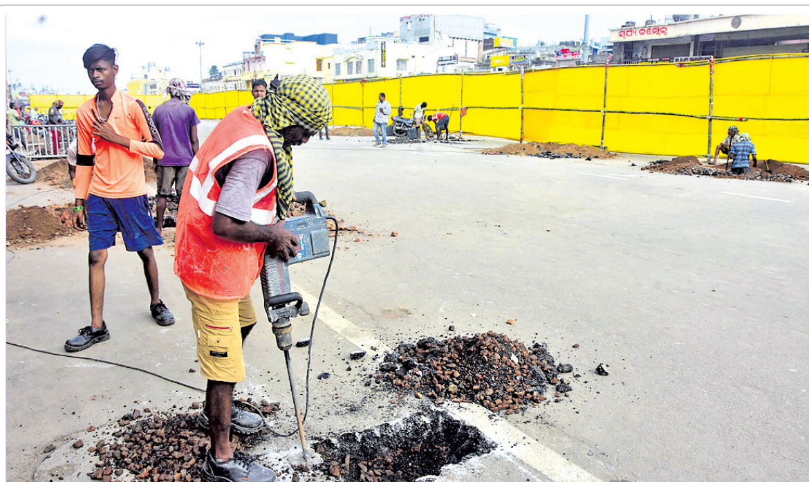
FOR HASSLE-FREE DARSHAN: Workers initiate process to set up air-conditioned tensile fabric structure on Grand Road in Puri that would help streamline queue management system for devotees visiting Srimandir, Friday
