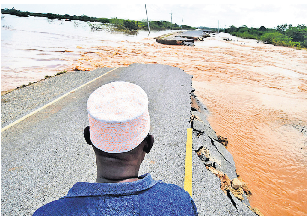
Members of the public view a section of the main Garsen-Lamu road at Gamba village which was swept away by heavy floods, in Gamba, Kenya
