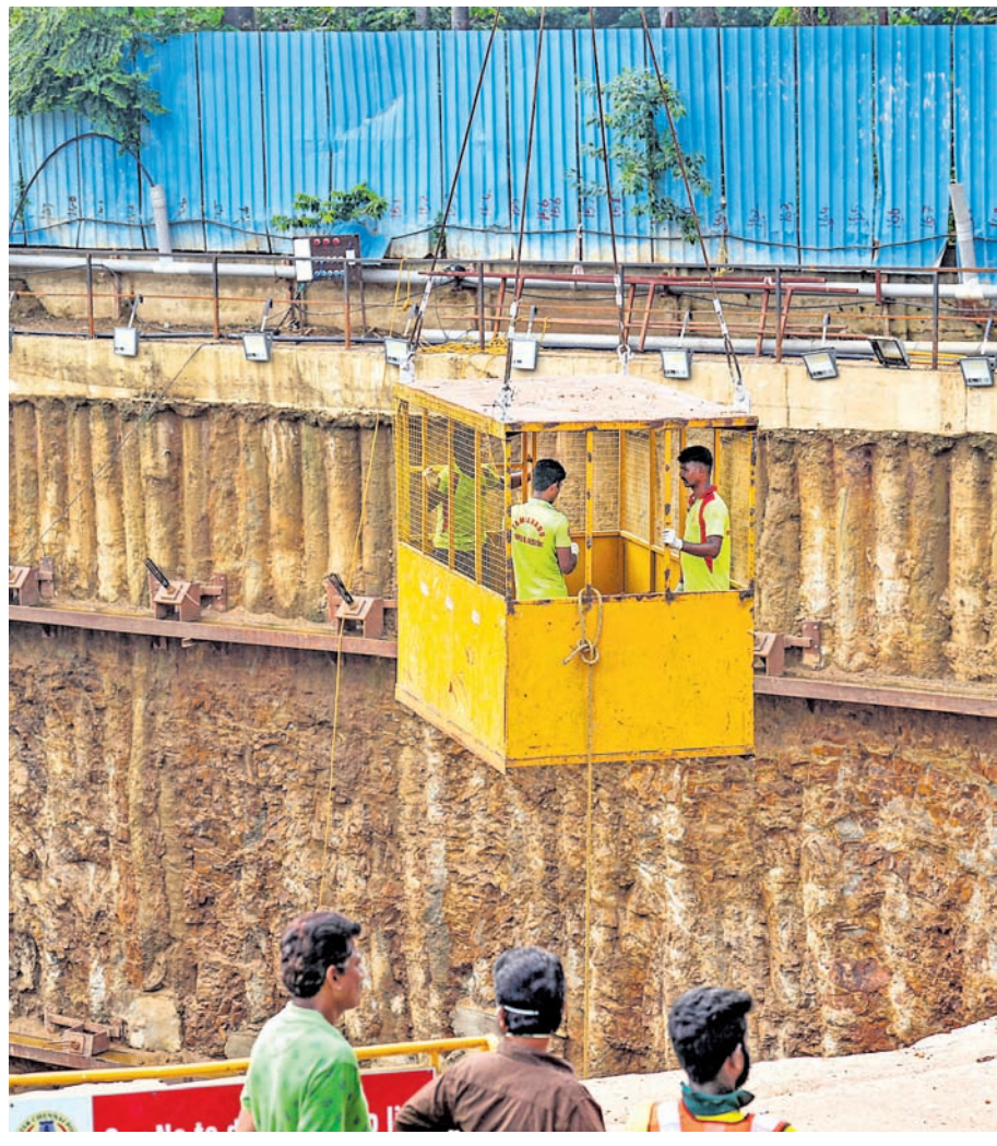
Rescue operation underway after the structure caved in at a construction site in which two people are feared dead, on the Five Furlong Road-Velachery Main Road junction, in rain-hit Chennai
