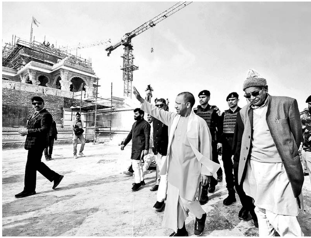
UP Chief Minister Yogi Adityanath inspects the construction work of Ram temple in Ayodhya, Thursday
