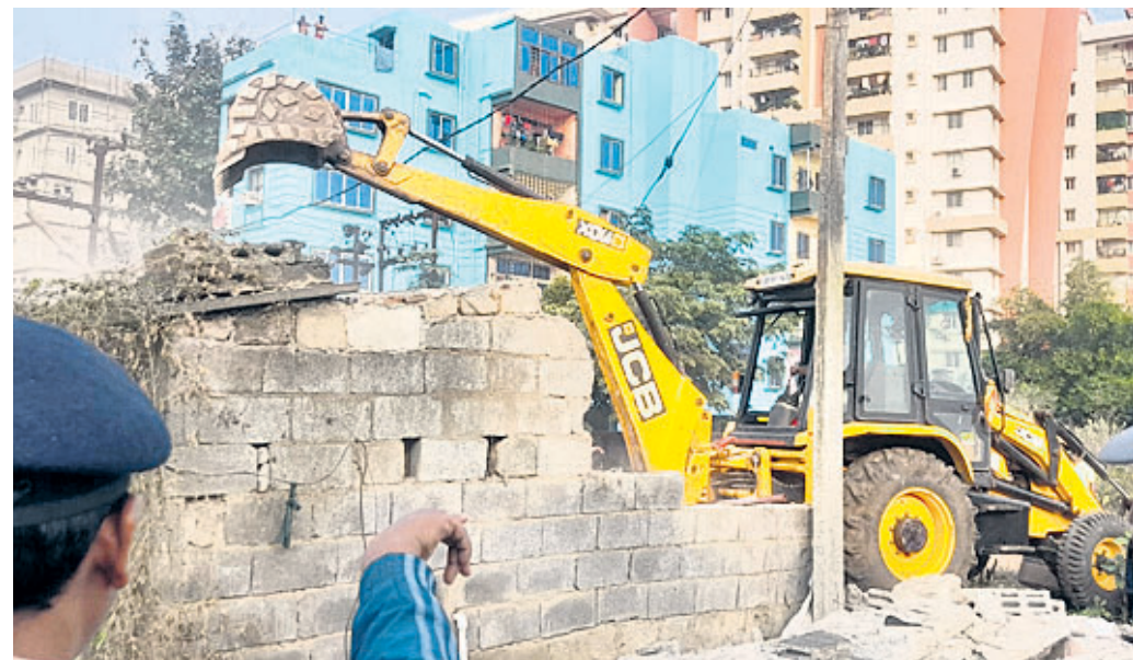
EVICTION DRIVE: An excavator deployed by BDA razing down unauthorised constructions in Chandrasekharpur area of Bhubaneswar, Tuesday
