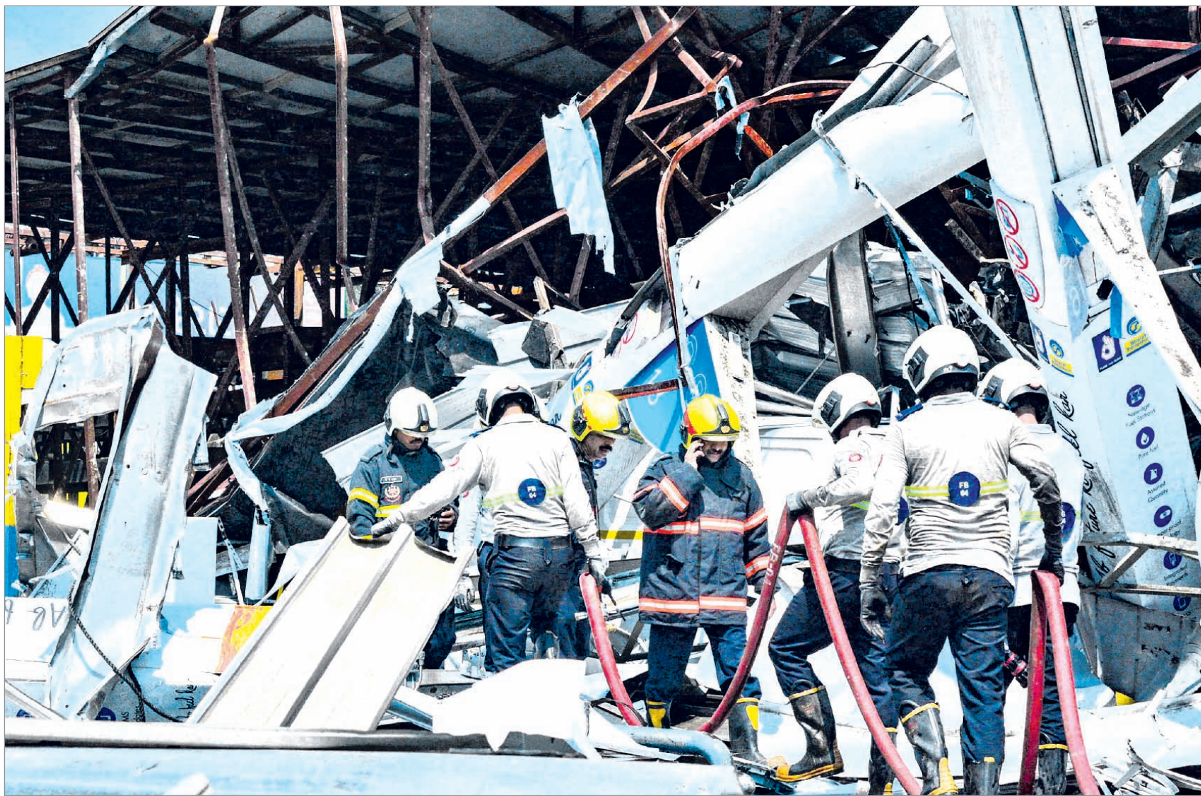
RESCUE OPS: Fire Brigade personnel seen cooling the site of the hoarding collapse at Ghatkopar, in Mumbai, Tuesday. At least 14 persons were killed and 76 others injured Monday night when a 100-foot tall illegal billboard fell on a petrol pump
