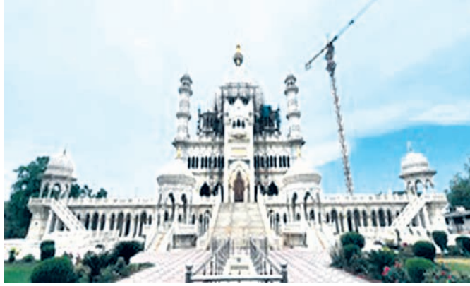
Resting on a foundation of 52 wells, the 193-foot tall structure, all in white marble from
