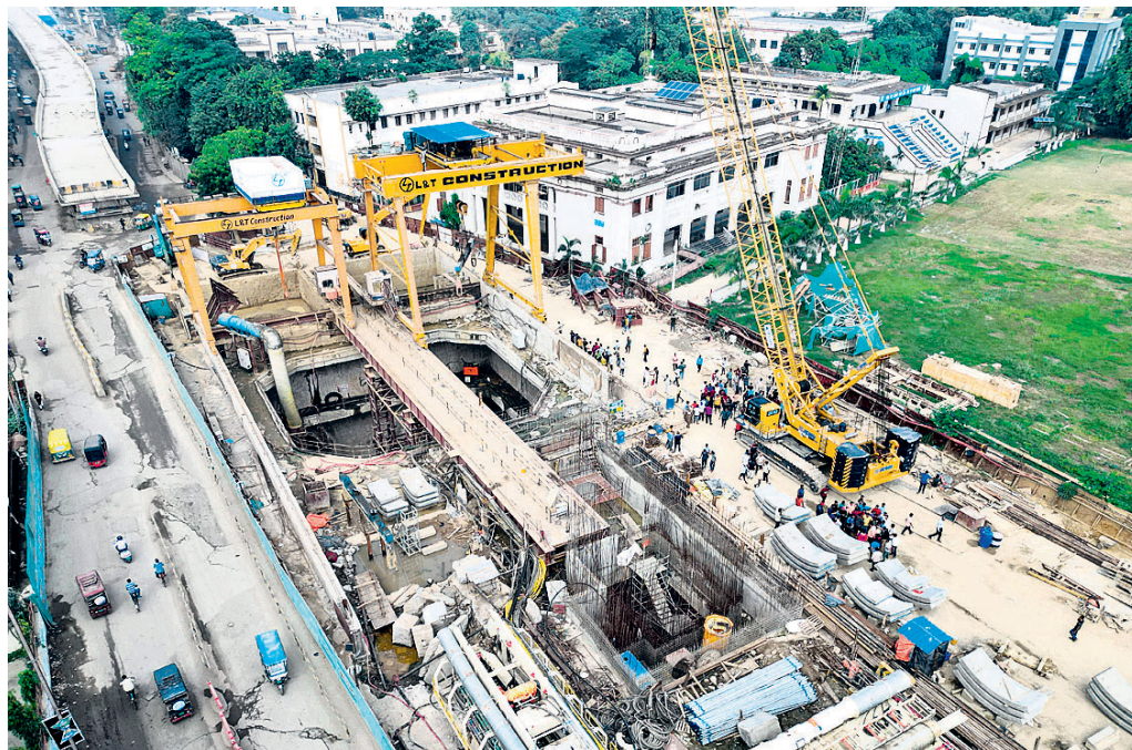
The Patna Metro tunnel construction site where two people died and many others injured after they were buried under soil, at Patna Science College NIT more, in Patna, Bihar
