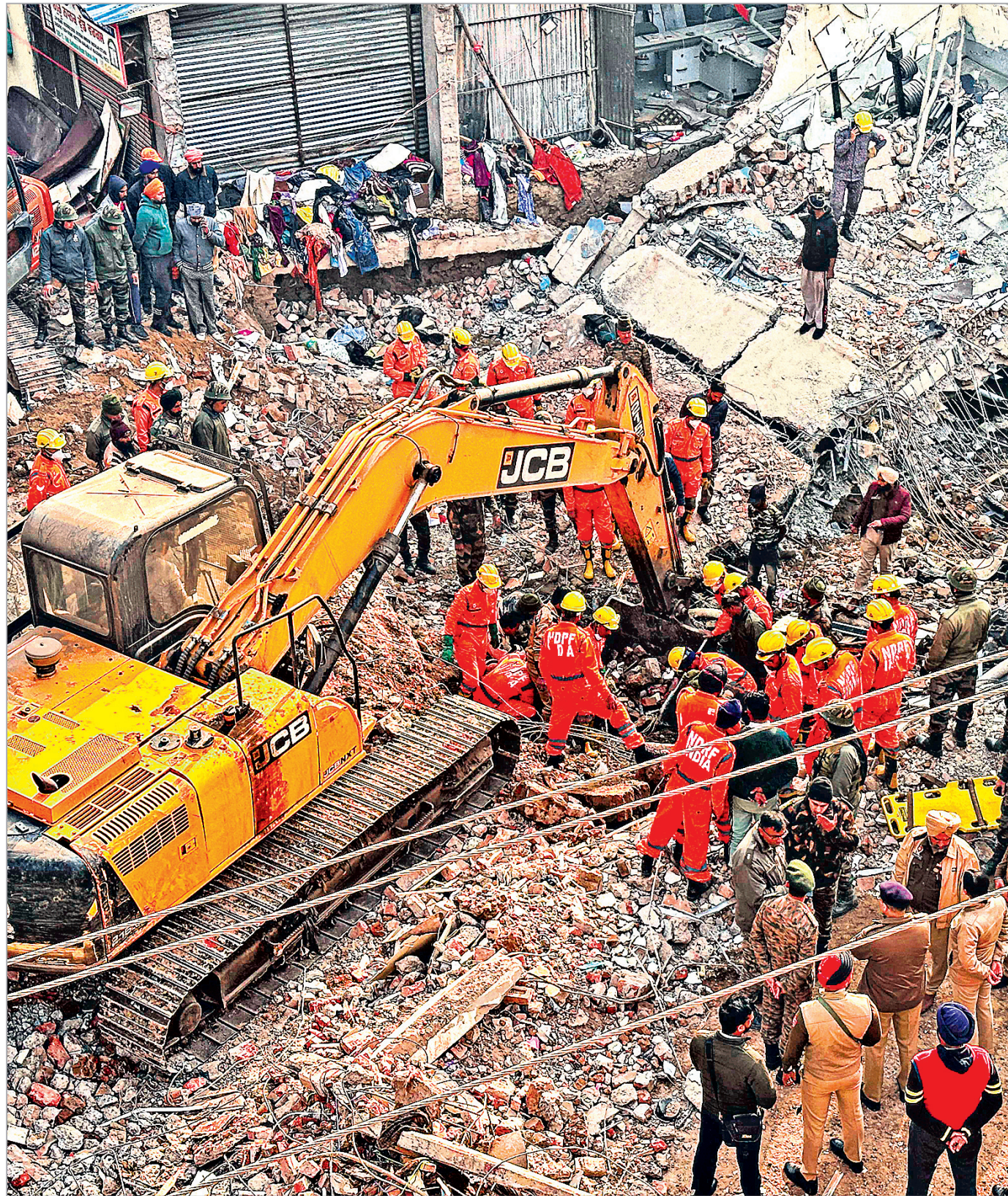
RUBBLE TROUBLE: Rescue operation continues after a multi-storey building collapsed Saturday evening, at Sohana village in Punjab's Mohali district, Sunday. At least two people were killed in the incident while several others are feared trapped under the debris, according to officials. PTI PHOTO
