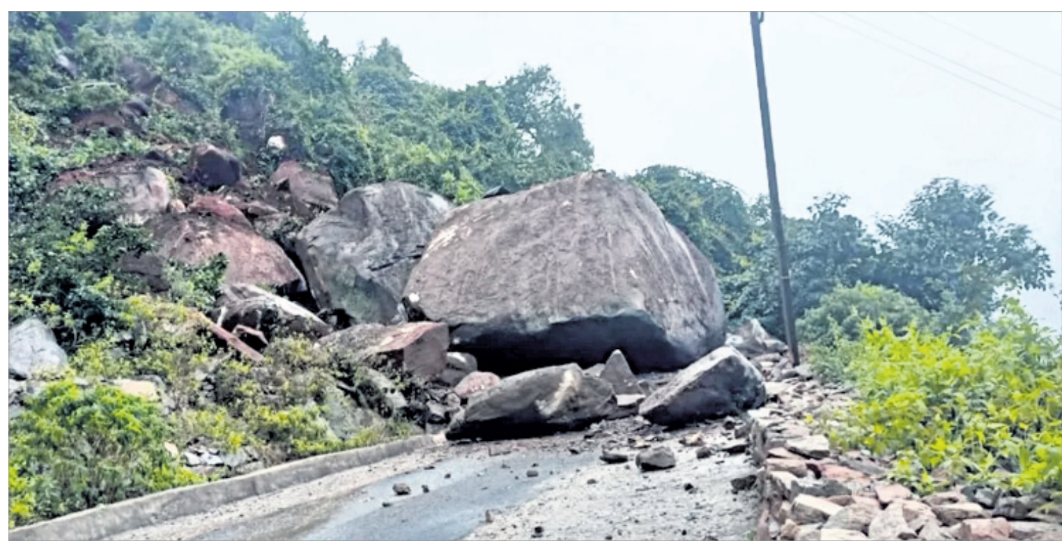
CYCLONE IMPACT: Communications on National Highway-326(A) passing through Anagha panchayat in R Udayagiri block of Gajapati district was disrupted following cyclonic storm ‘Montha’ induced landslide on the adjoining hill Tuesday
