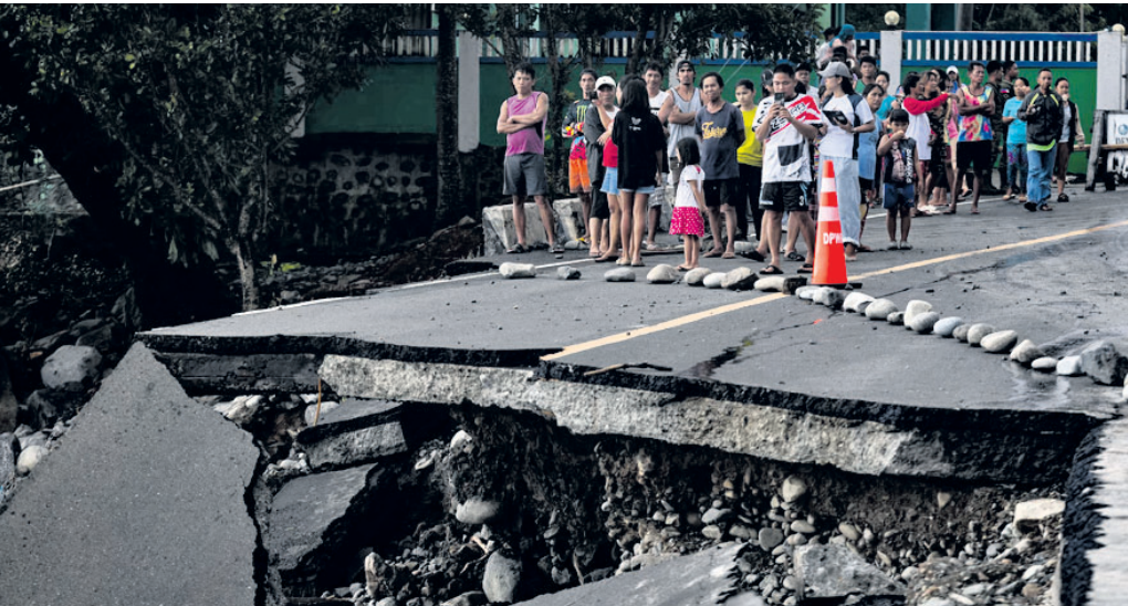
People stand near a wrecked part of the Baler-Casiguran road a day after Typhoon Fung-wong made landfall in Dipaculao, Aurora, Philippines
