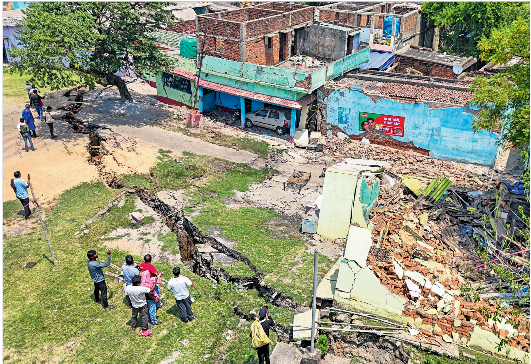
NATURE'S FURY: Residents gather near damaged houses following a land subsidence at Tandabari village, in Dhanbad, Friday. The incident, reported late Thursday night, damaged several houses and prompted evacuation of affected families.
